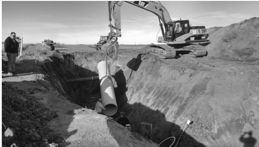
Irrigation employees from the Holdrege office use heavy equipment to install a new pipeline providing a new water delivery point to the Funk Lagoon.
