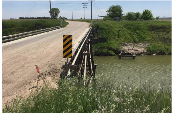
The Johnson Lake inlet bridge was closed due to safety reasons by Gosper County. Central signed an agreement to build a replacement bridge.
