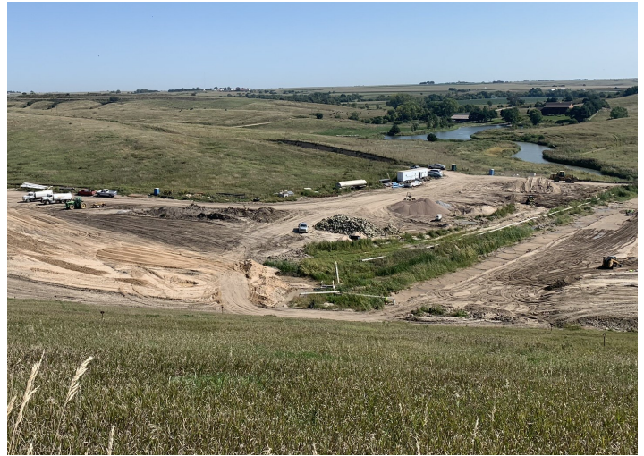
Construction crews complete the installation of the seepage mitigation system on north side of Elwood Dam
