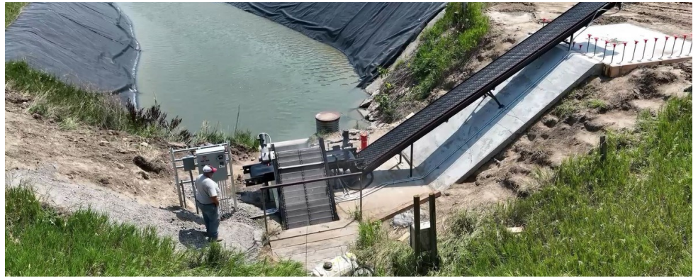
An overhead view of the new conveyor system at the inlet of the lined E67 Canal.
