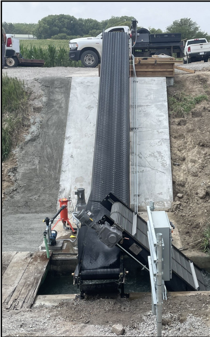
The new water screen and conveyor system removes trash before entering the E67 Canal
